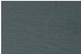
The joint has been damaged throughout by UV radiation.
